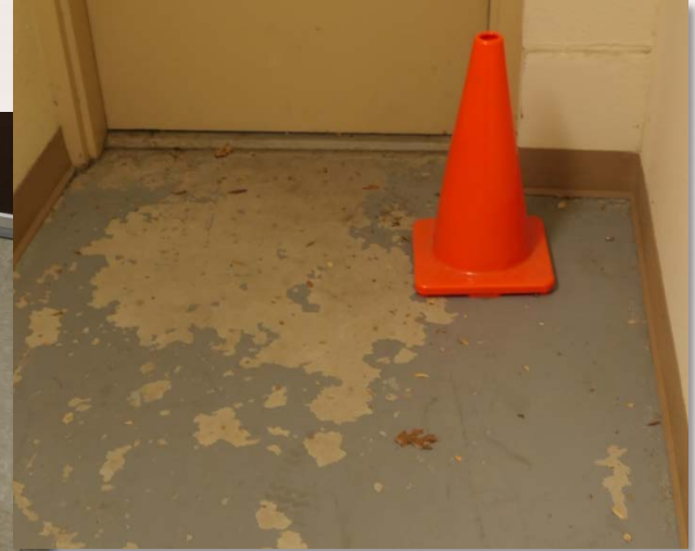
WORN AND FLAKING FLOOR COATING
