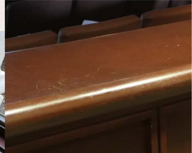
SCRATCHED AND DAMAGED DOORS AND TRIM
