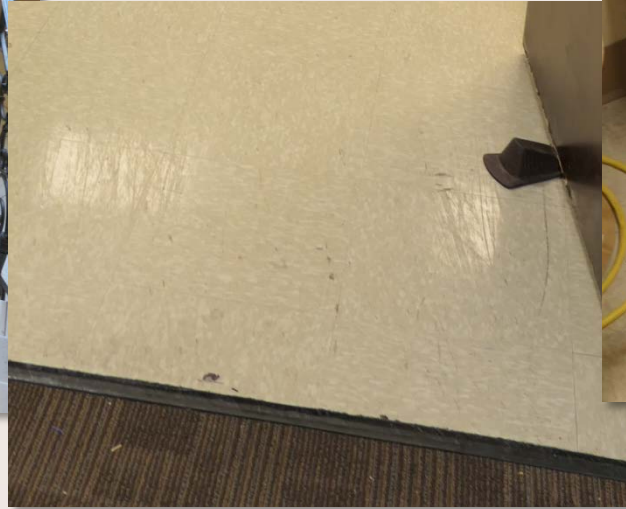
SCRATCHED AND PEELING FLOORING TILE
