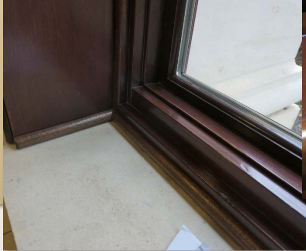
FADED WOOD STAINED TRIM AND WINDOW SILLS
