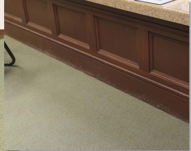
SCUFFED AND SCRATCHED MILLWORK
