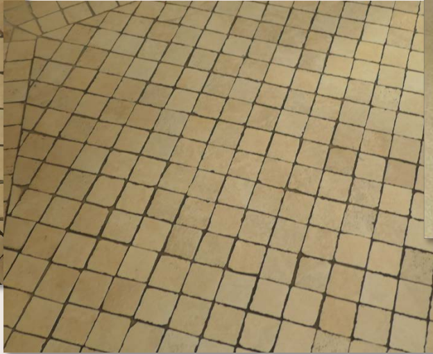
WORN TILE FINISH
