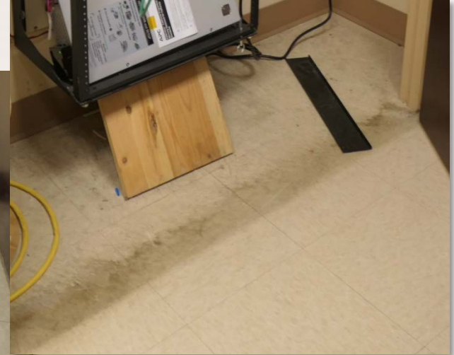
STAINED AND DISCOLORED FLOORING
