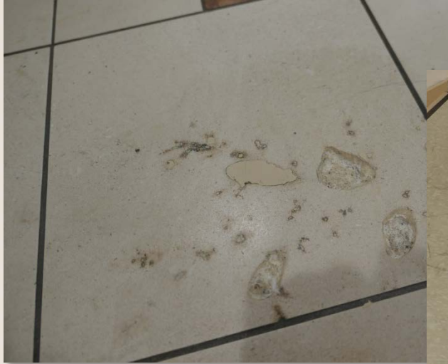
DETERIORATING STONE TILE
