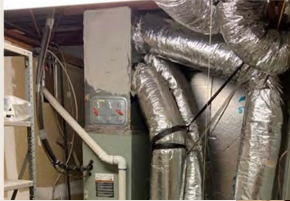
Existing HVAC System
