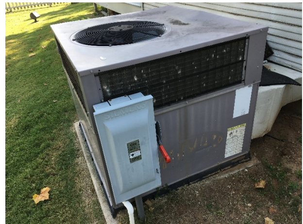
Existing HVAC unit adjacent to north façade.
