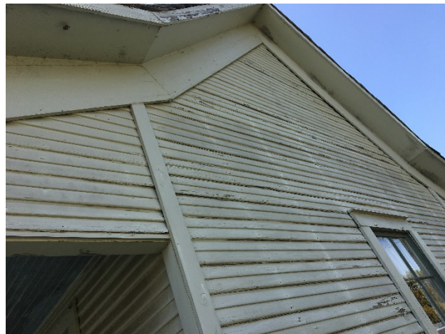
Existing siding and trim (repair required)
