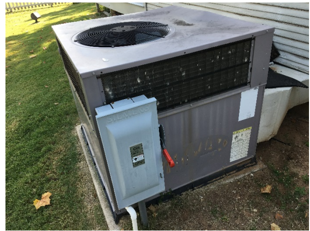
Existing HVAC unit adjacent to north façade.
