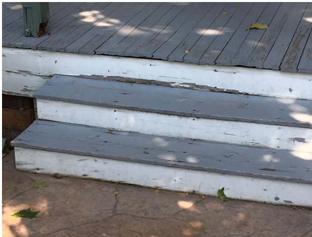
Existing porch and steps (repair required)
