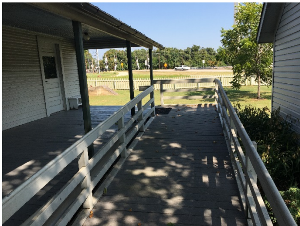
Existing ramp (violates current ADA standards for slope, railing, and landing size)
