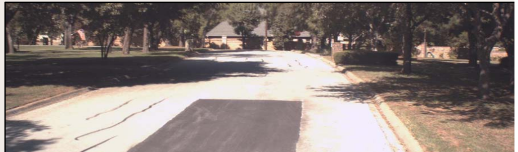
Poor/Very Poor/Serious PCI (11 to 55)
