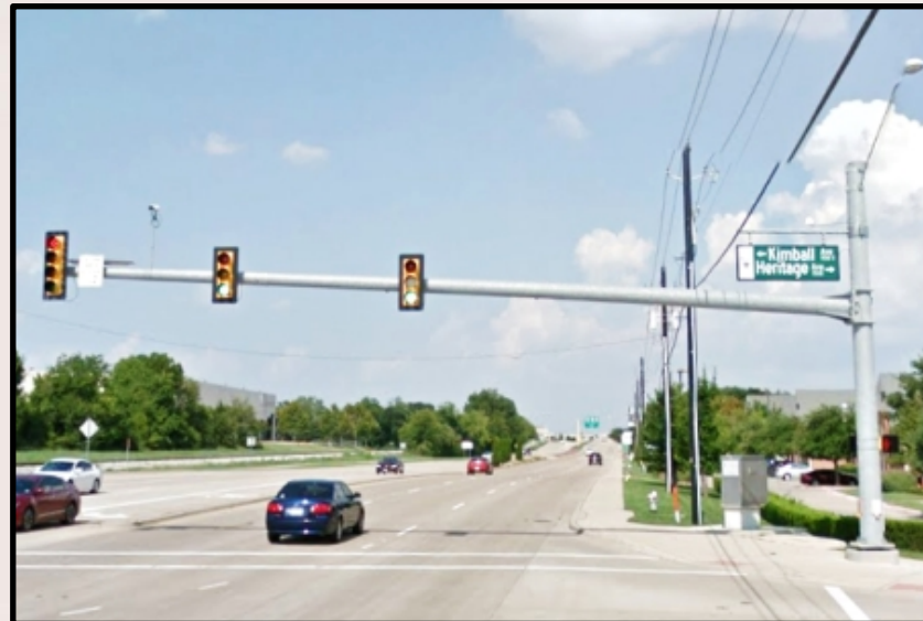
Standard Signal Poles
