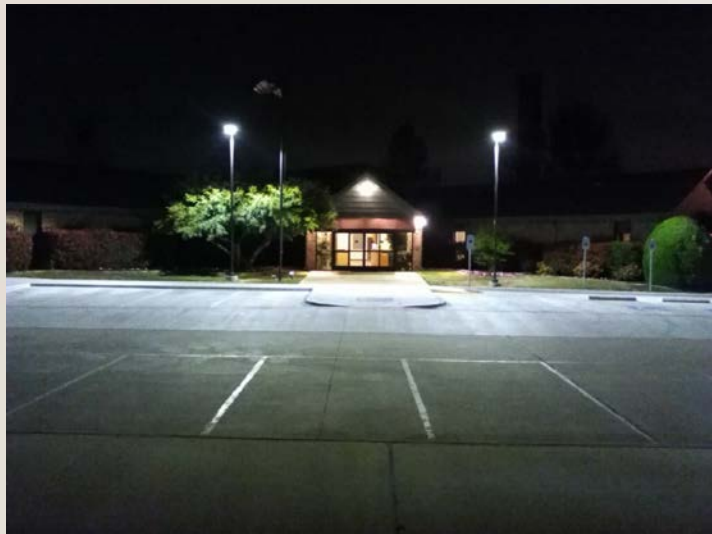
Parking Lot Lights
