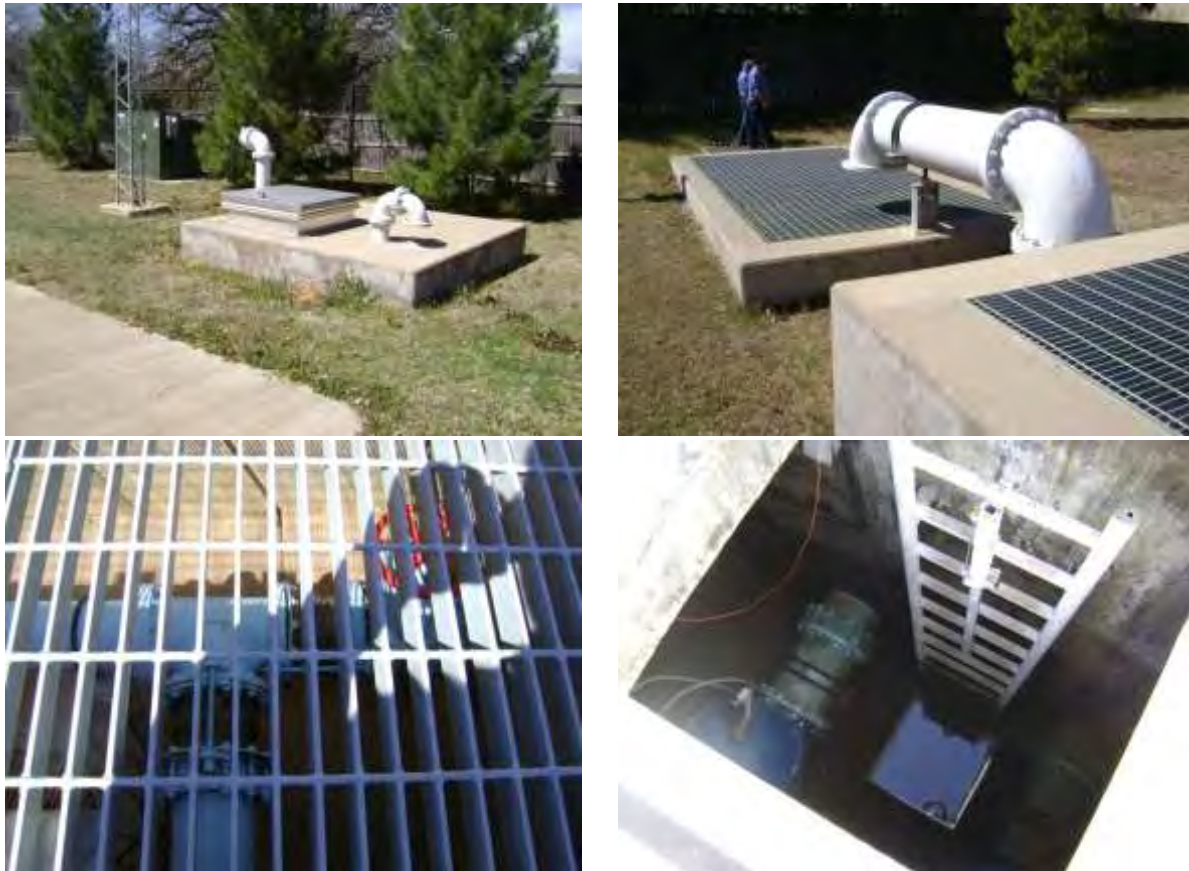
Figure 20: L.D. Lockett PS Vaults
