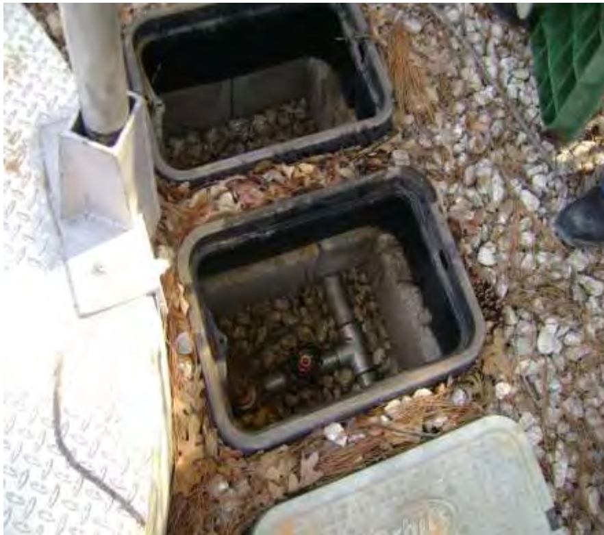
Figure 9: Valve Boxes at Overland Trail Lift Station
