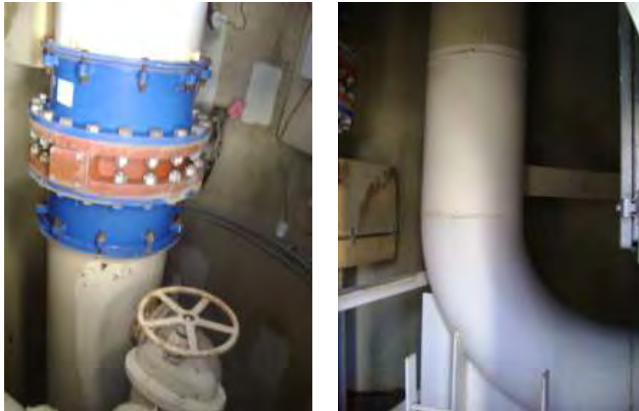
Figure 26: Interior Piping at Bransford Elevated Storage Tank
