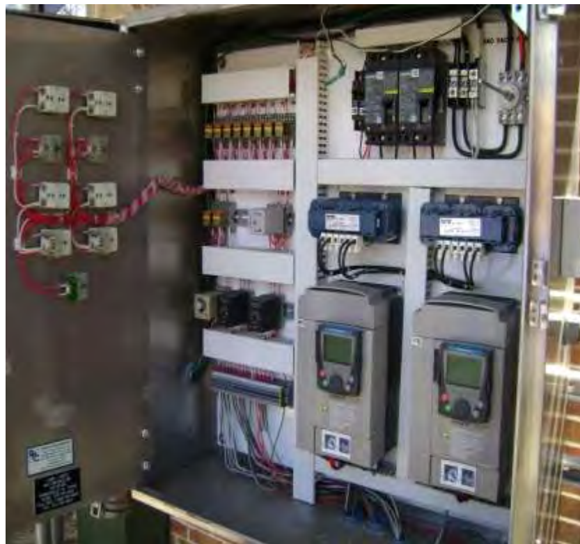
Figure 18: Interior of Control Panel at Reserve Lift Station
