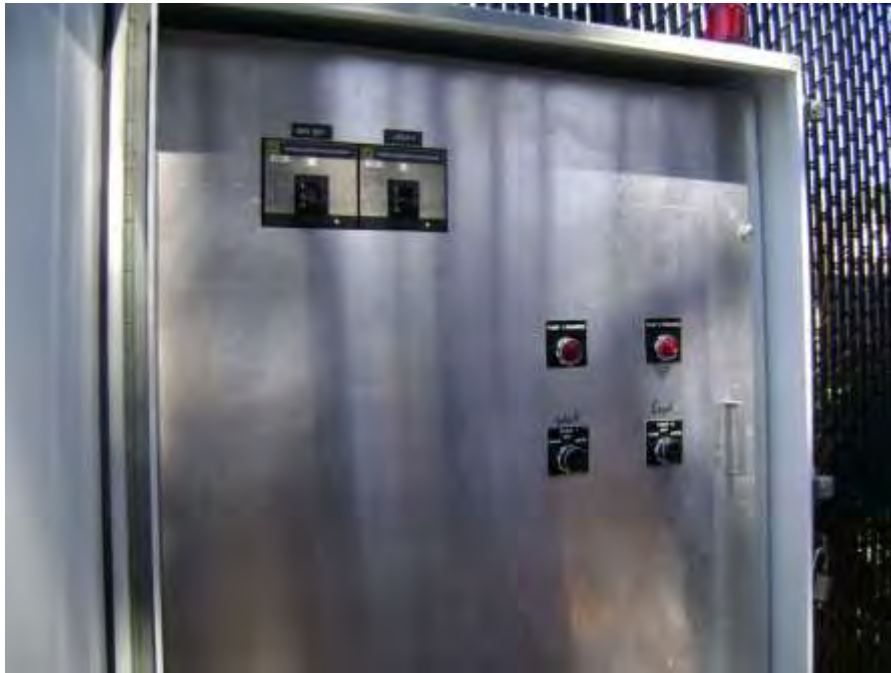
Figure 8: Control Panel at Overland Trail Lift Station
