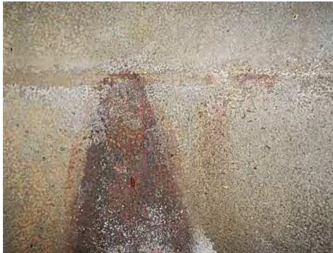
Figure 29: Manhole 1640 Defect - Evidence of Groundwater Intrusion
