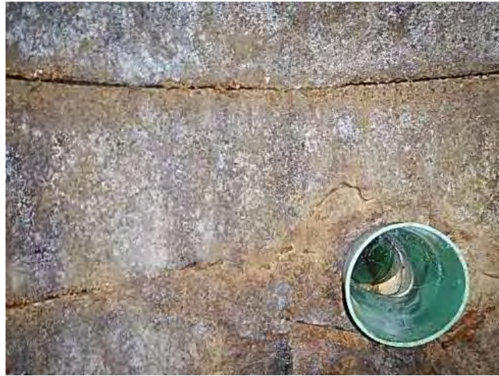
Figure 30: Manhole 1640 Light Defect – Defective Joint
