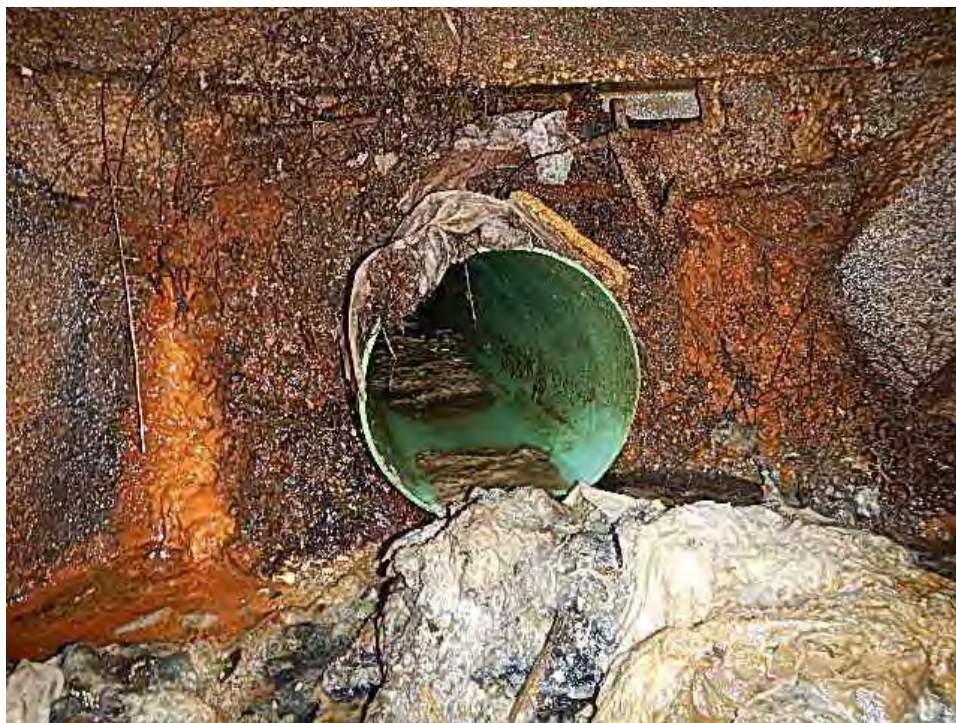
Figure 31: Manhole 2158 Severe Defect - Priority 1 Debris and Bad Pipe Seal
