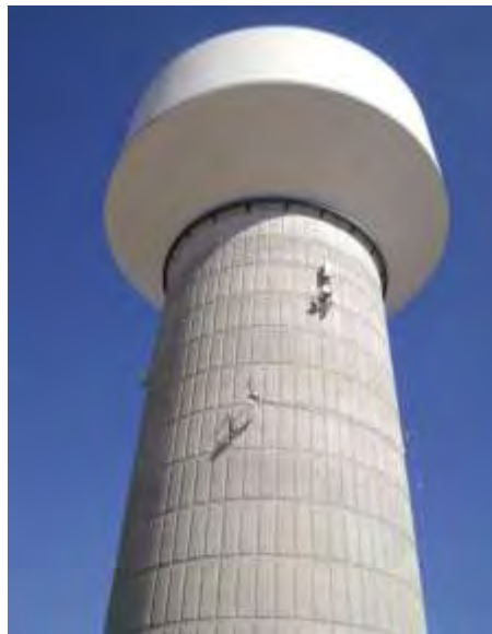
Figure 30: McPherson Elevated Tank
