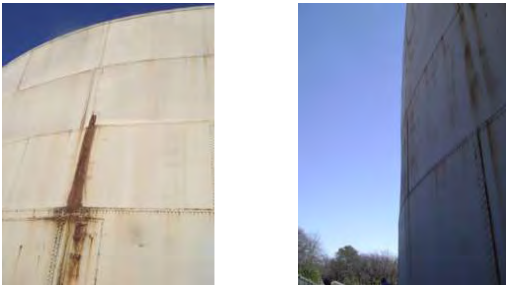
Figure 15: Corrosion on Overland Trail Ground Storage Tank
