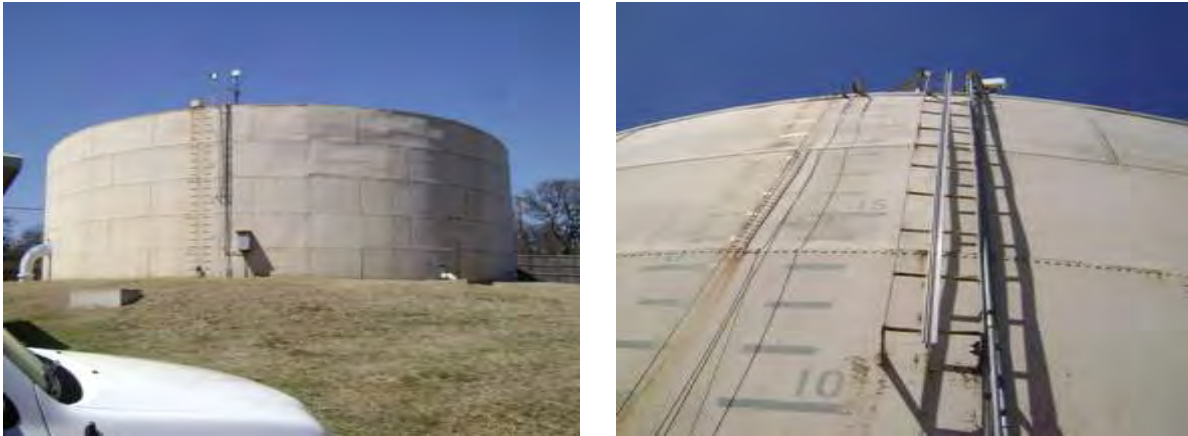
Figure 14: Evidence of Overland Trail Ground Storage Tank Buckling
