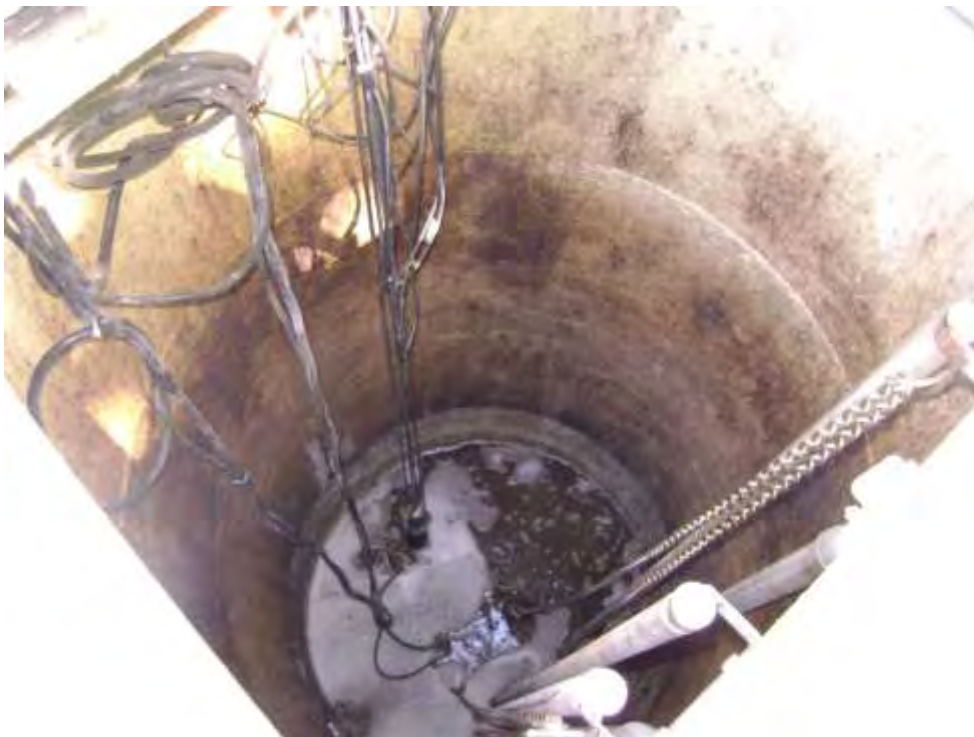
Figure 11: Pump Controls at Overland Trails Lift Station
