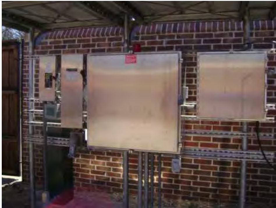
Figure 17: Mounted Control Panels at Reserve Lift Station
