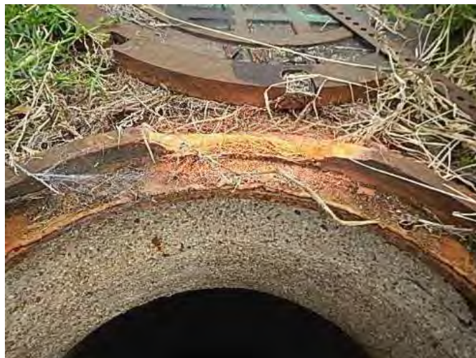
Figure 27: Manhole 1640 Light Defect- Broken Frame
