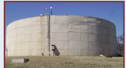
The Overland Trail Ground Storage Tank is in poor physical condition. The Master Plan recommends decommissioning this tank.
