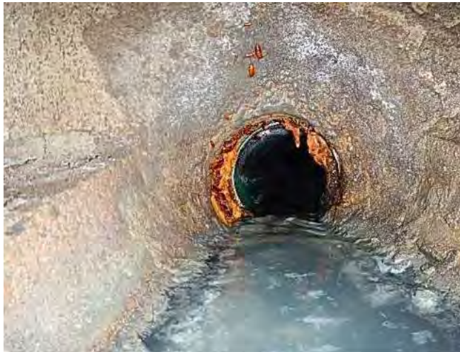
Figure 28: Manhole 1640 Moderate Defect – Bad Pipe Seal
