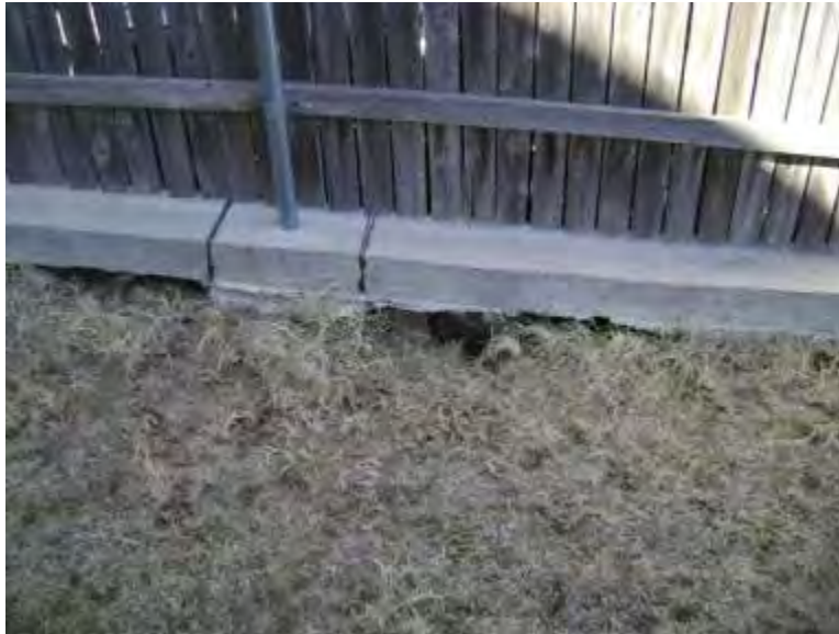
Figure 9: Erosion at Overland Trail Northern Fence
