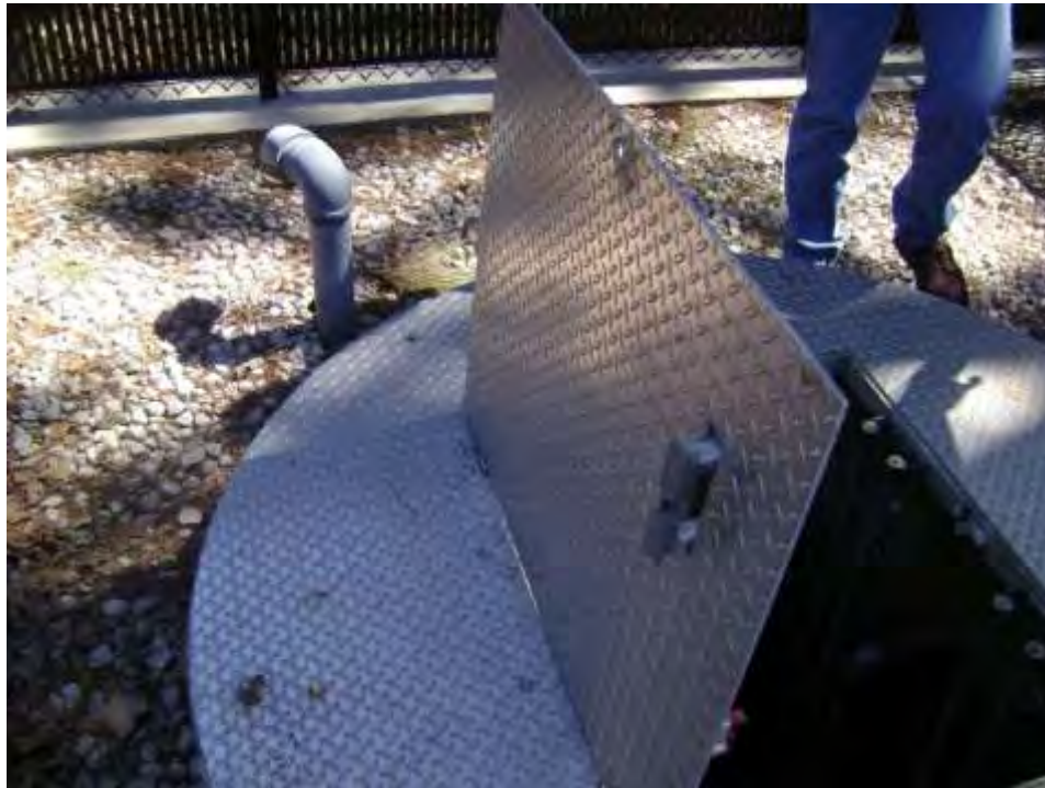
Figure 10: Wet Well Vent at Overland Trail Lift Station
