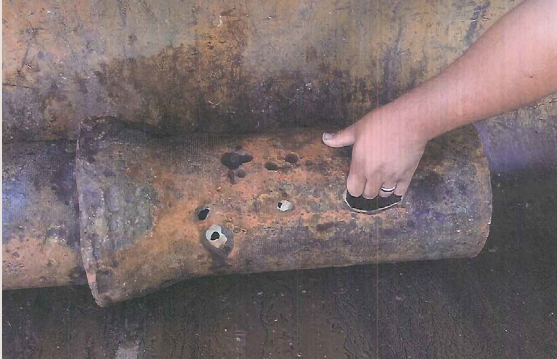
December Water Main Break at the 99 Cent Store
