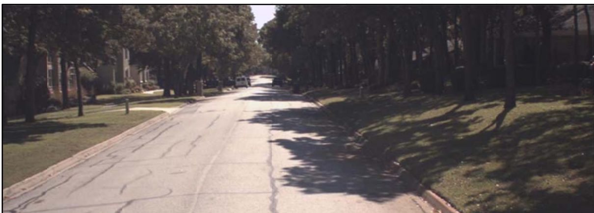
Figure 13 – Street with Yellow/Fair PCI (50 to 70)
