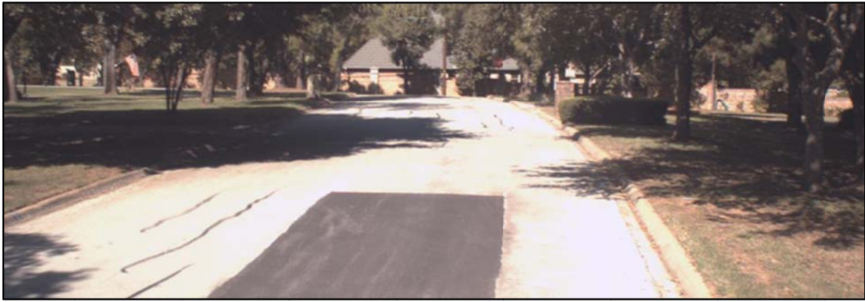
Figure 14 – Street with Red /Poor PCI (0 to 50)
