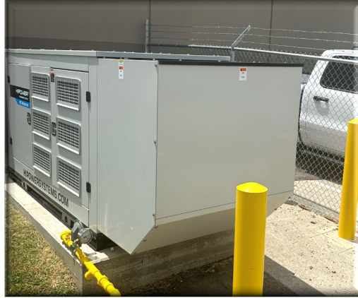
Public Works Emergency Generator Contract Award $291,869
