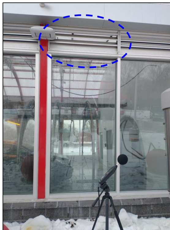
Figure 11 – Photo of the Tommy's Express Car Wash with an open damper circled.
